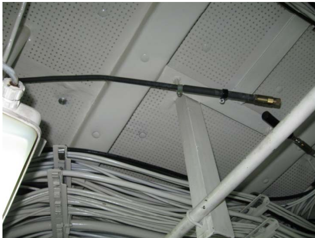
OEM stub antenna, disconnected for removal
