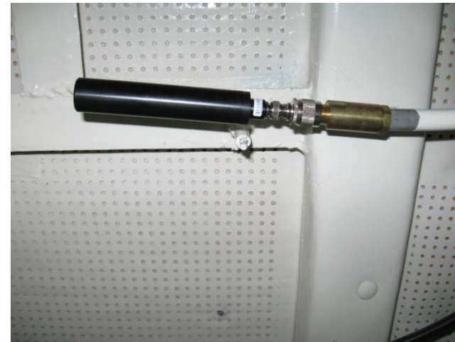
SFRT Antenna, installed and in service
